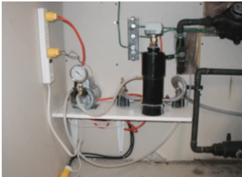
FIGURE 5 – ROTRONIC TEMPERATURE/HUMIDITY TRANSMITTER (INCOMING SEWER AIR)
